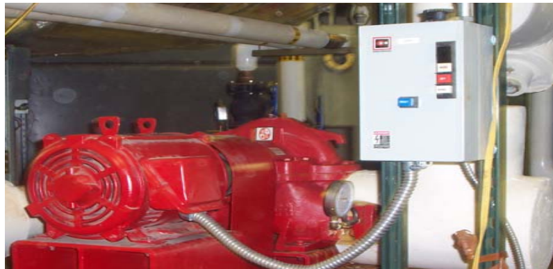
Heating and Air Conditioning Plant
